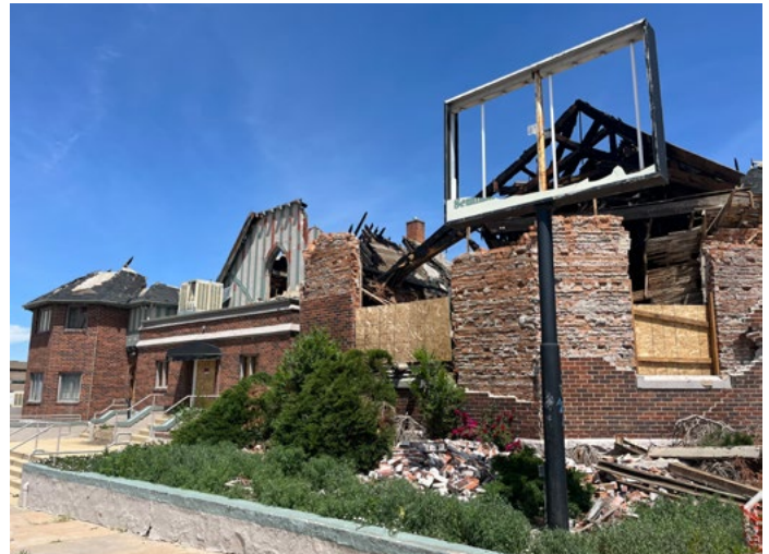
Asbestos Survey of Historic Albany Building After Fire Damage, Pueblo, CO
