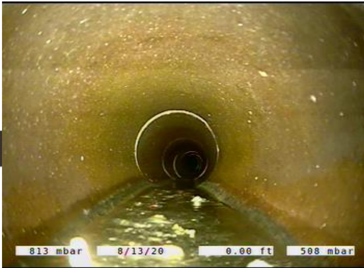
BROKEN VOID VISIBLE
