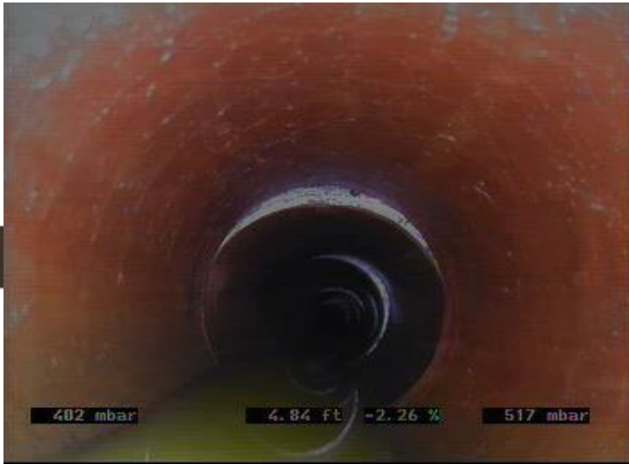
HOLE SOIL VISIBLE AND FRACTURED PIPE
