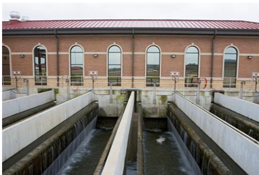
Figure 10. Example Severn Trent Denite® Filters
